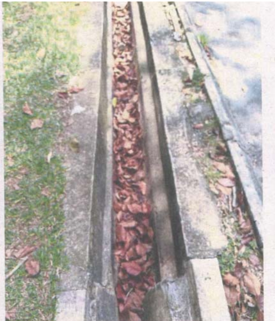
A drain filled with dried leaves appears to be poorly maintained by the cleaning contractor.
